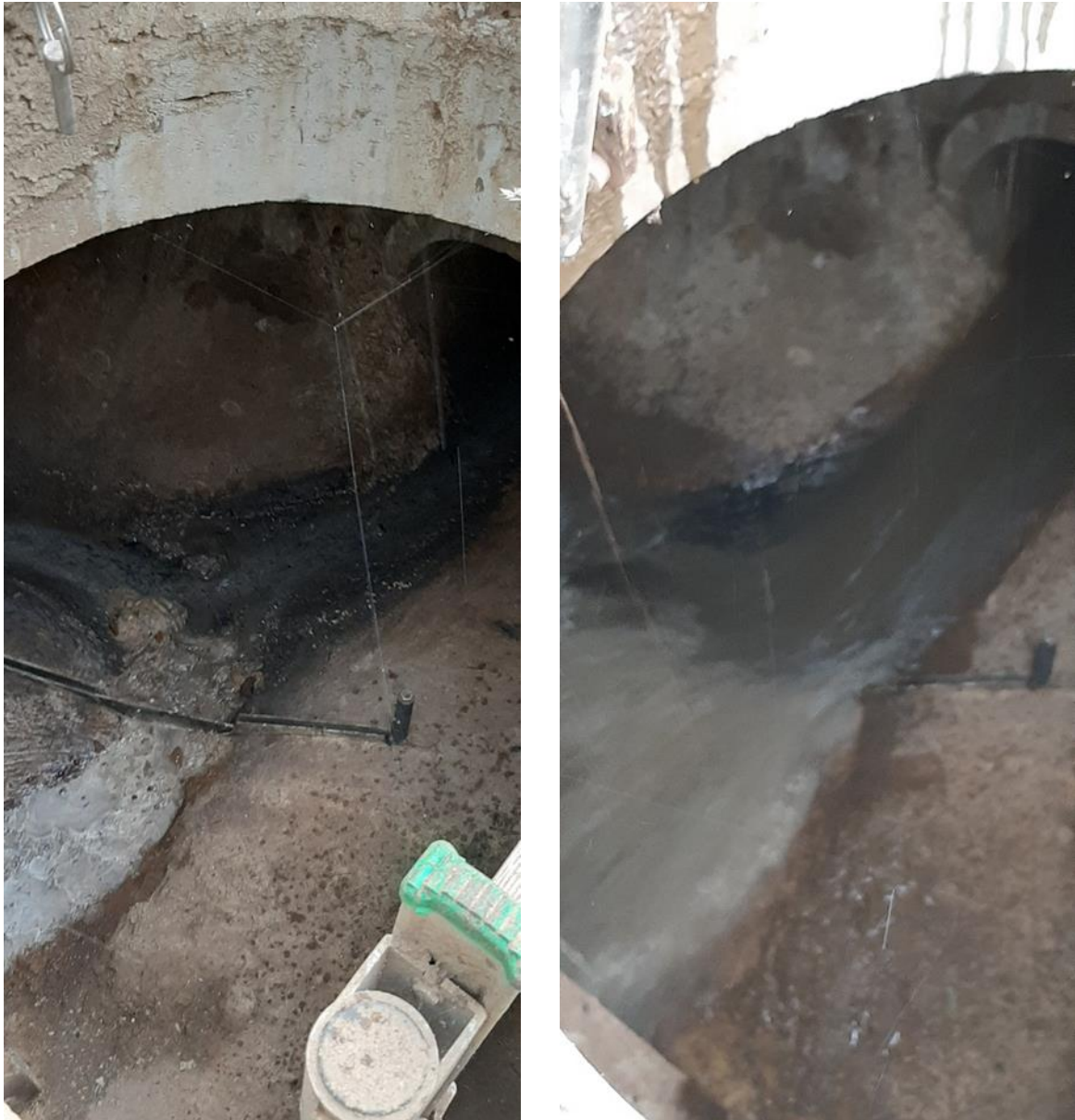
Figure 22. Sewer and threshold before (left) and after (right) rainfall.
